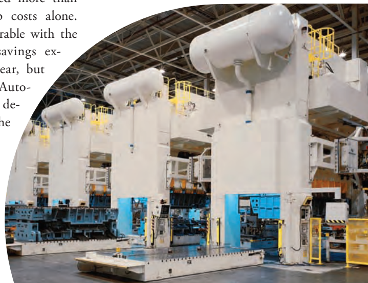
The Allen-Bradley GuardLogix controller helps International Automation reduce installation time and increase efficiency.
